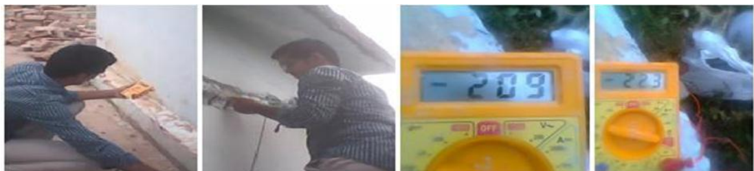
Fig 4.1 Half Cell Potential Difference test being conducted on the Ration Shop building
