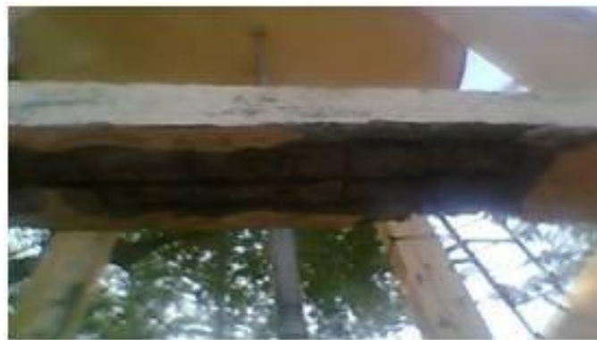
Fig.3.3 Image of the Spalled Brace of the Water Tank
